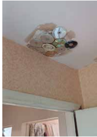
Fig. 5 Vernacular methods of sealing a ceiling leak using old compact discs. Amguema, 2024. Photo: Gavriil Malyshhev.
